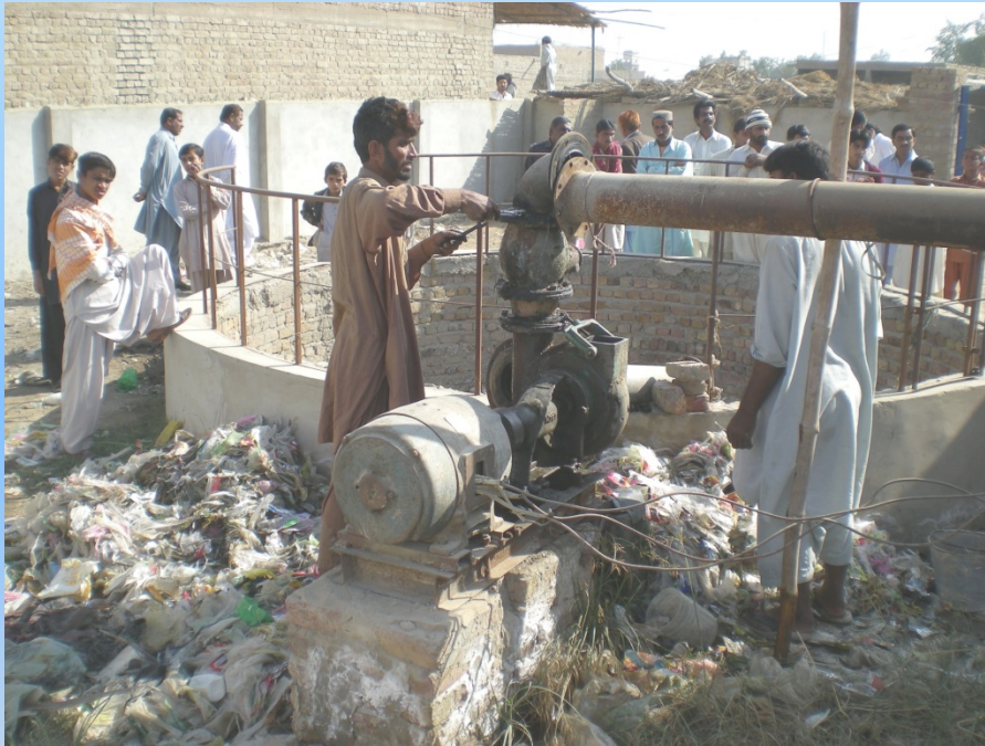
Larkana, Pakistan – single pump, high suction lift, poorly aligned. Needs frequent repair
