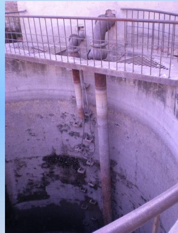
Sialkot, Pakistan. Wet well - dry well arrangement failed. Replaced by pump with high suction lift
